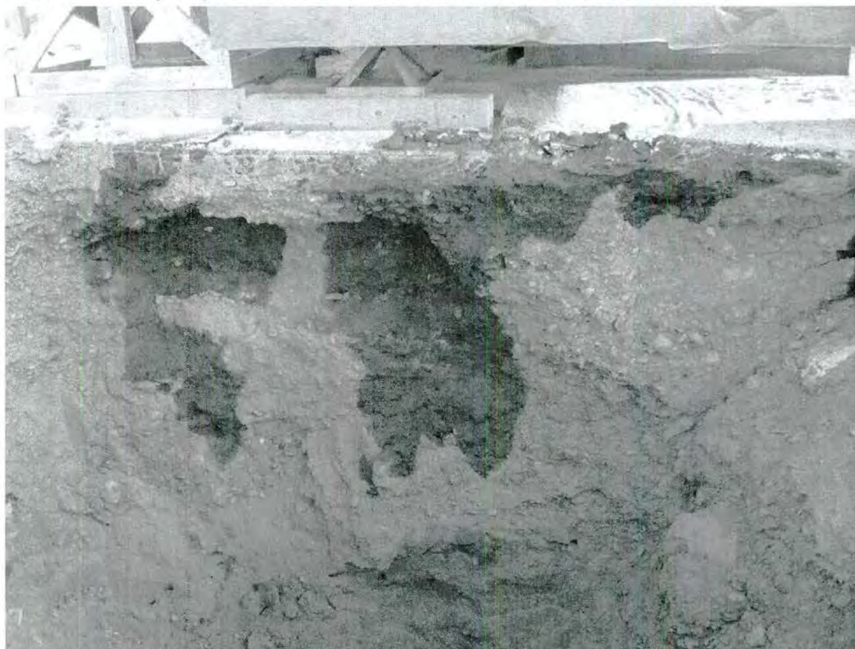
Photo 15 – Mobility of hydrocarbons on west side excavation wall after scarification work
