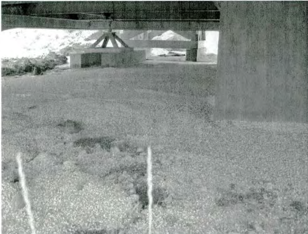
Photos 5 and 6 – Surface soils below building covered with sorbent materials
