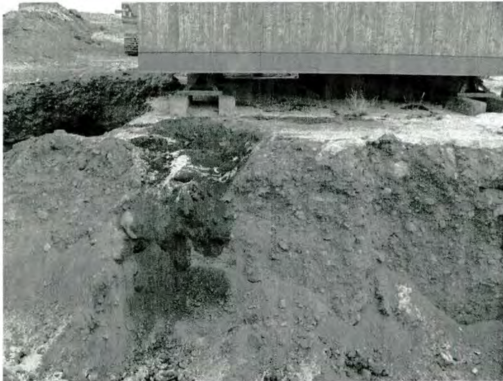
Photos 13 and 14 – Extra scarification work on the south side of the station
