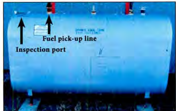
5.3 Double-wall 1,135 litre (250 gallon) steel heating oil tank. Note the inspection port on the top left end of the fuel tank.
