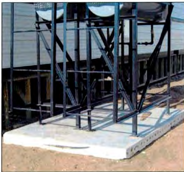
4.4d A twin tank installation firmly secured to a full concrete pad. This provides a solid foundation.
