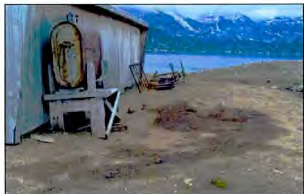
4.9 Excessive ground staining from a poorly installed and maintained oil tank.
