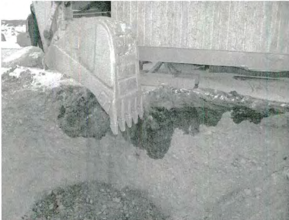
Photos 11 and 12 – Extra scarification work on the west side of the station
