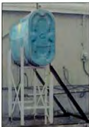
4.4c Note that owner has stabilized the base of his oil tank by lengthening the horizontal support members on the side of the tank where the fuel delivery ladder is located, and adding steel struts at a 45-degree angle to provide greater stability.
