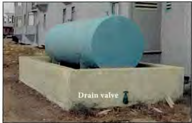
4.11 4,550 litre (1000 gallon) tank with a concrete berm. Note that the drain valve is not fitted with a lock or chain and thus can be tampered with.
